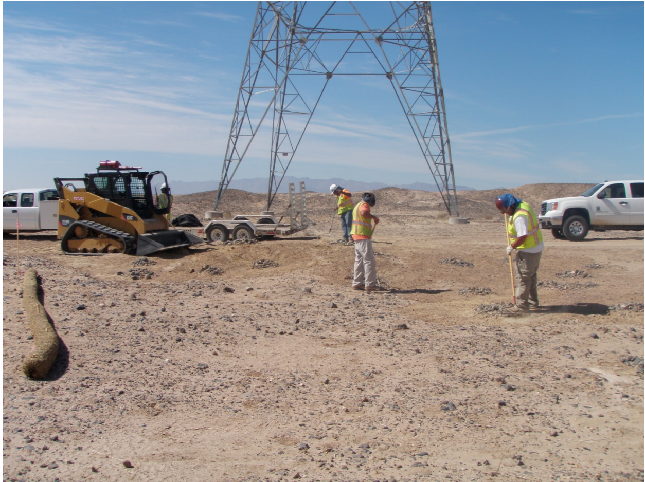
Crew salvaging desert pavement for restoration after Project completion. Photo courtesy of Jennifer Kaminsky.
