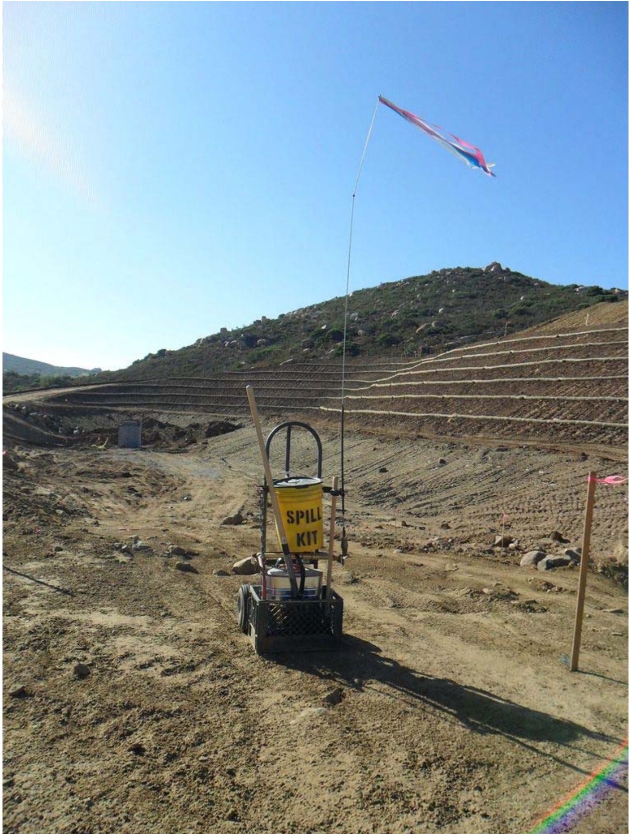
Mobile fire/spill response cart used when a fire box is not near work activities. Photo by Mark Meridith.
